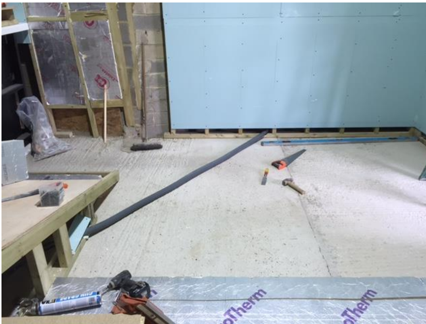
Preparation works prior to install included wooden ramp ready for covering with Altro flooring.
