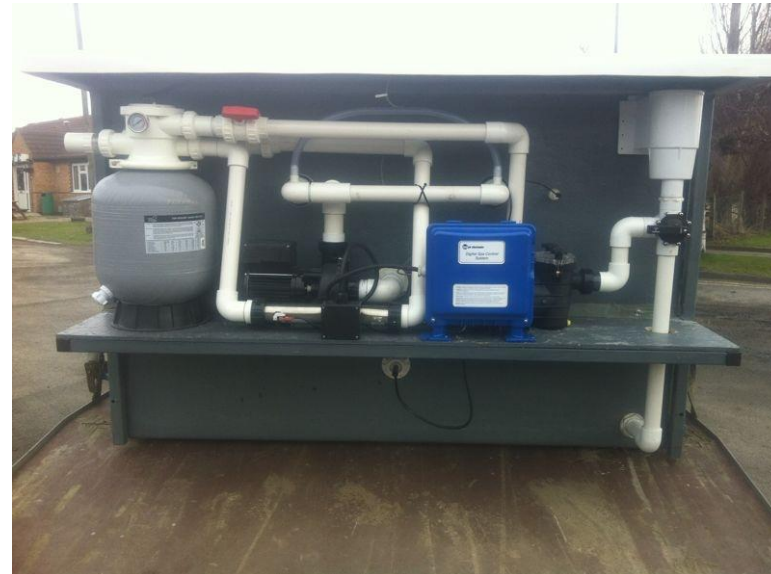
Built-In Plant Example
