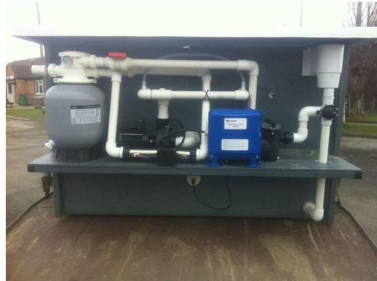
Built-In Plant Example
