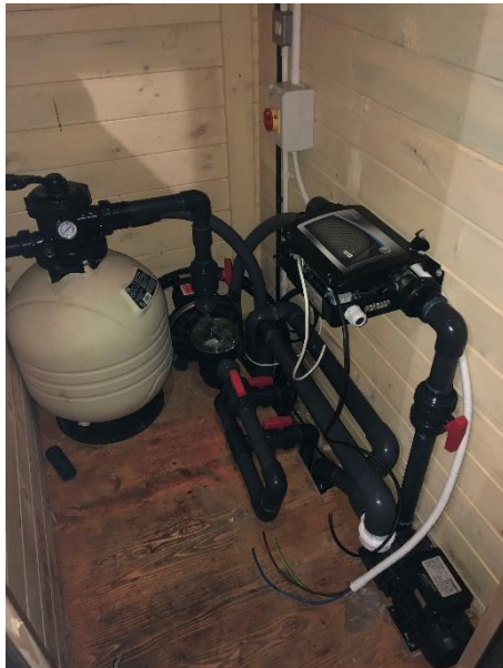
Plant Room Example
